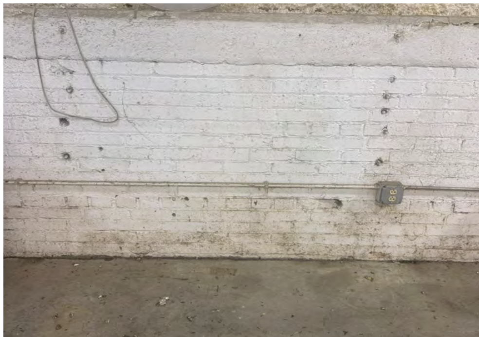
3. View of LBP on brick wall along east side of Diesel Shop (#7)
