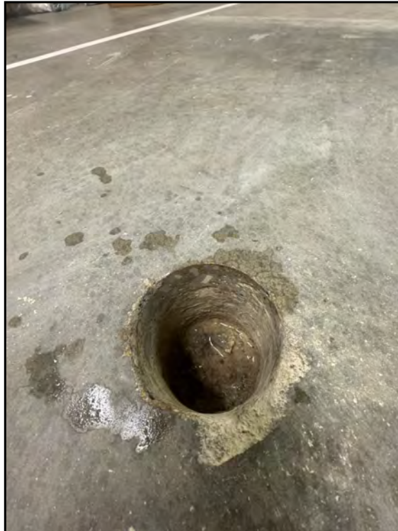
19: View of CF-ST-1 in low bay/small transformer area.
