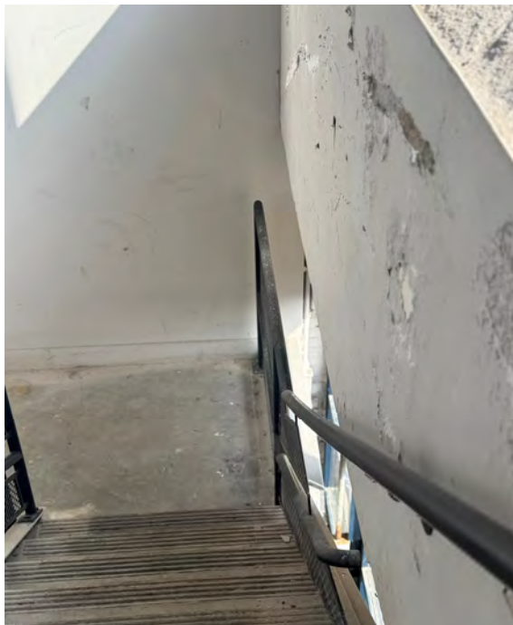
11. View of LBP on stair rail in office tower stairwells (#123)
