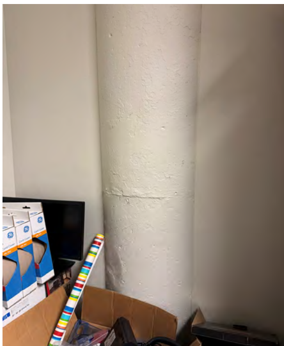
12. View of LBP on concrete pillar in the 5th floor office (#147)
