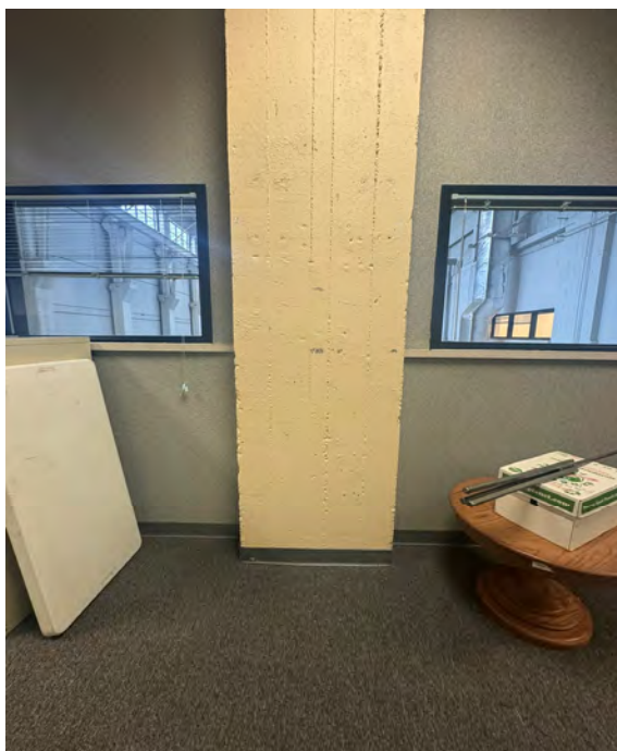
16. View of LBP on concrete column in 2nd floor office (#191)
