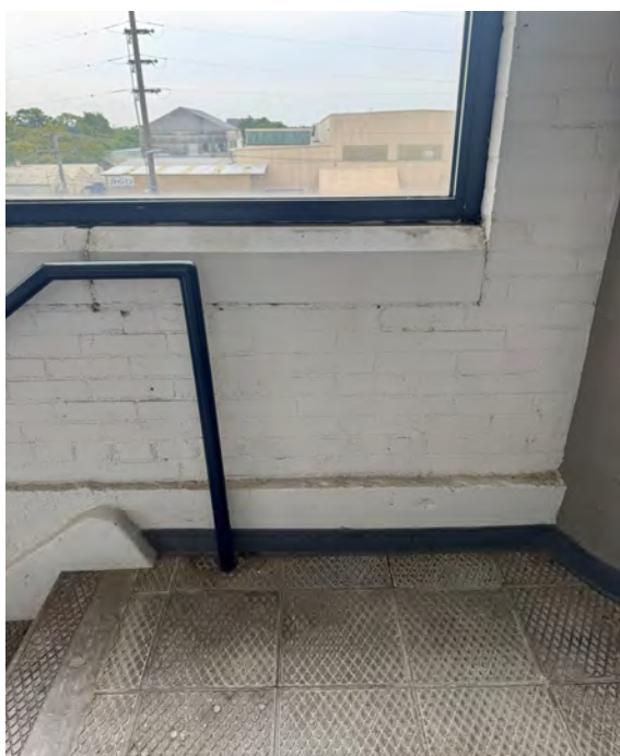
12. View of LBP on brick wall and concrete trim in office stairwell (#161, 162)
