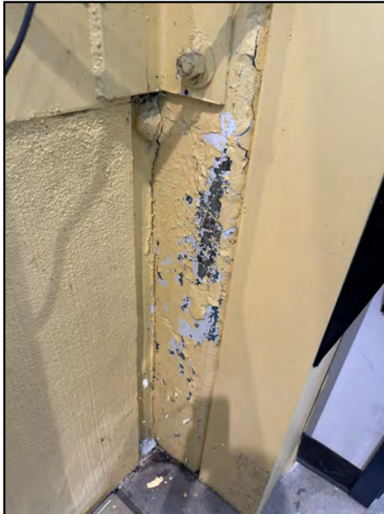
37: View of paint on concrete columns along west wall of high bay (PC-HB-5-3).
