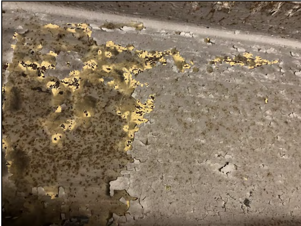
27: View of paint on ceilings/cross beams in low bay (PC-LB-2-3).
