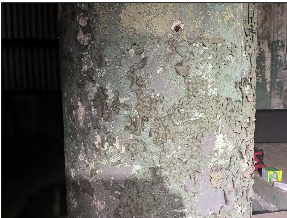
44: View of concrete pillar paint in north tower (PC-NT-12-1).
