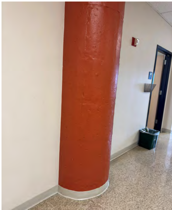
13. View of LBP on concrete pillar in 3rd floor office (#158)
