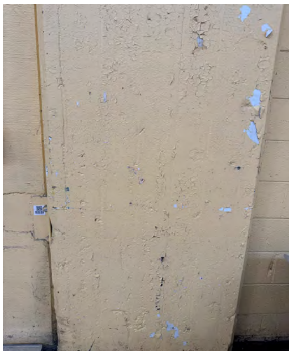
10. View of concrete column with LBP in High Bay along west wall (#88)
